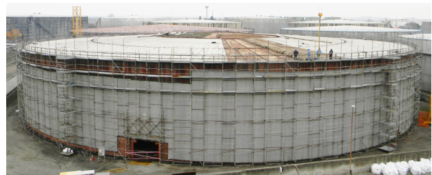
BEFORE. An aged oil storage tank in a refinery had a heavily corroded roof and urgently needed repair.
