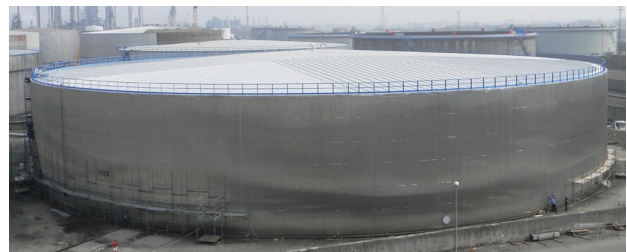
AFTER. The tank roof newly insulated with a 30 mm insulation solution and long lasting corrosion protection.
